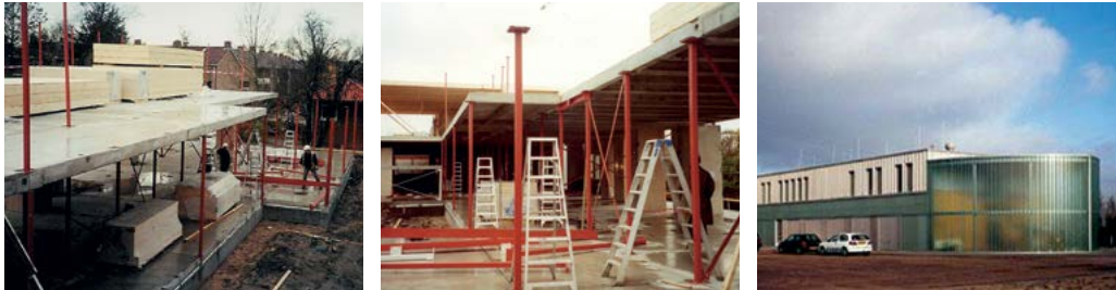
Figure 4.5. The modular UCB construction system under construction and the right is finished
